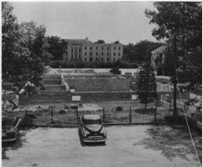
PROGRESS — Photo above, taken at the end of July, shows Activities Building foundation well under way. Since picture was taken, steel beams and trusses have been installed, basic plumbing and electrical lines completed, and the general area back-filled and graded.
